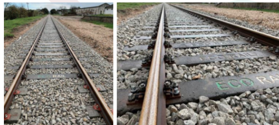
Completion of the works by end November 2020 - Section of the East Line where the Eco Rails were deployed.
